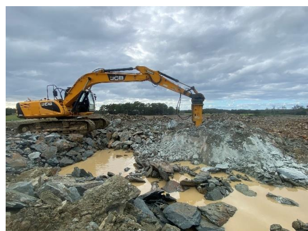
Bands of high strength rock in over-excavation area being broken up by hydraulic rock hammer.
